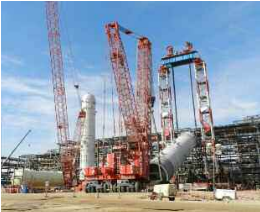
[Figure 8.6 – Reactor lifting Meg Project Singapore Foster Wheeler with Towers, Strand Jacks and Crane (Fagioli)]
