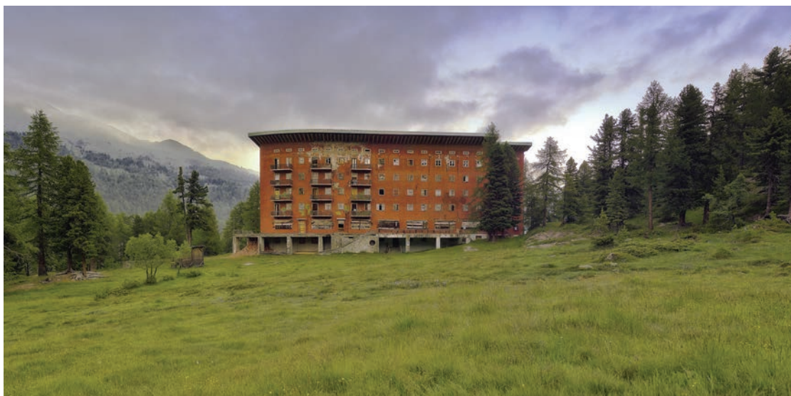
Fig. 3. The state of abandonment and neglect of the Sporthotel del Paradiso del Cevedale, Val Martello, designed by Gio Ponti with Antonio Fornaroli and Eugenio Soncini, 1935-1938. Photo by Alpes/Giorgio Dalvit ©
