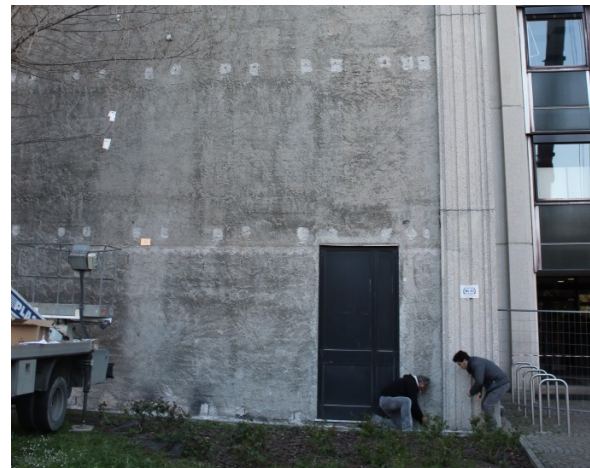
Fig. 10: individuation of the bubble and entire anchoring system set-up on the test façade.
