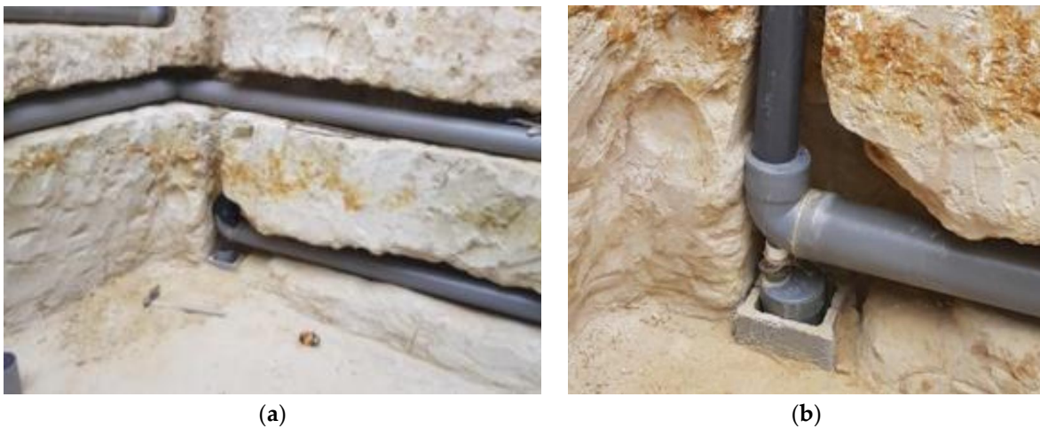
Figure 5. Photographic view of the installed EAHE system on site. (a) Pipeline within the gypsum soil. (b) Condensate drainage system.
