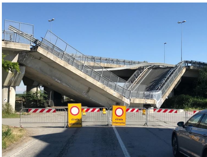
Figure 1 Collapse of Fossano bridge, 2017
