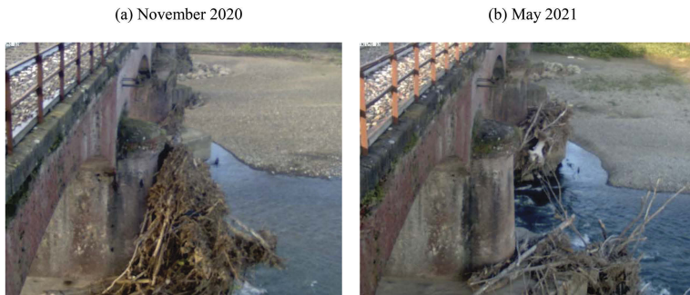
Figure 5. Pictures from the permanently installed cameras: (a) debris accumulation on P05 in November 2020 resulting from the important event of October 2020; (b) debris accumulation on P05 and P04 after the event of May 2021.
