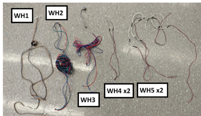
Fig. 120. All Wire Harnesses Running from Pellet Extruder to Ceiling Mount/DUET3 Controller.
