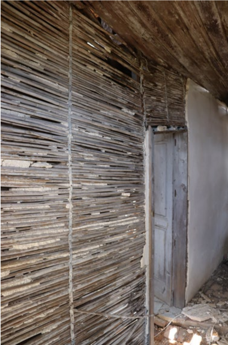
Figure 11. Ferruzzano Superiore. Remains of the lathwork in the internal partitions (photo C. Valiante, 2023).
