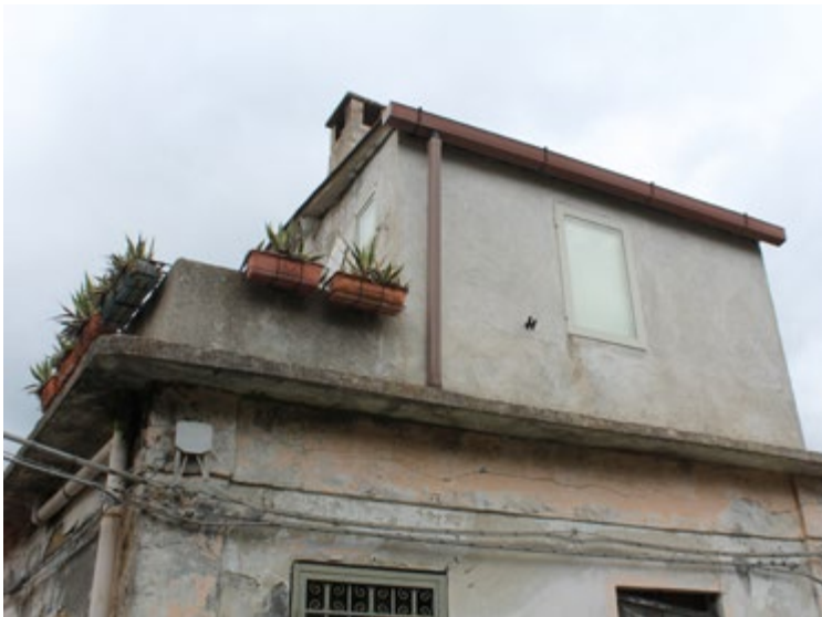
Figure 6. Ferruzzano, Reggio Calabria, pilot project. Elevations and additions (unit 305) (photo by the research group, 2023).
