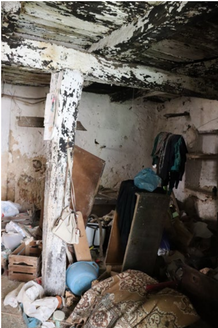
Figure 6. Characteristic presence of a central pillar in an abandoned building in via Pisacane (photo N. Sulfaro, 2023).
