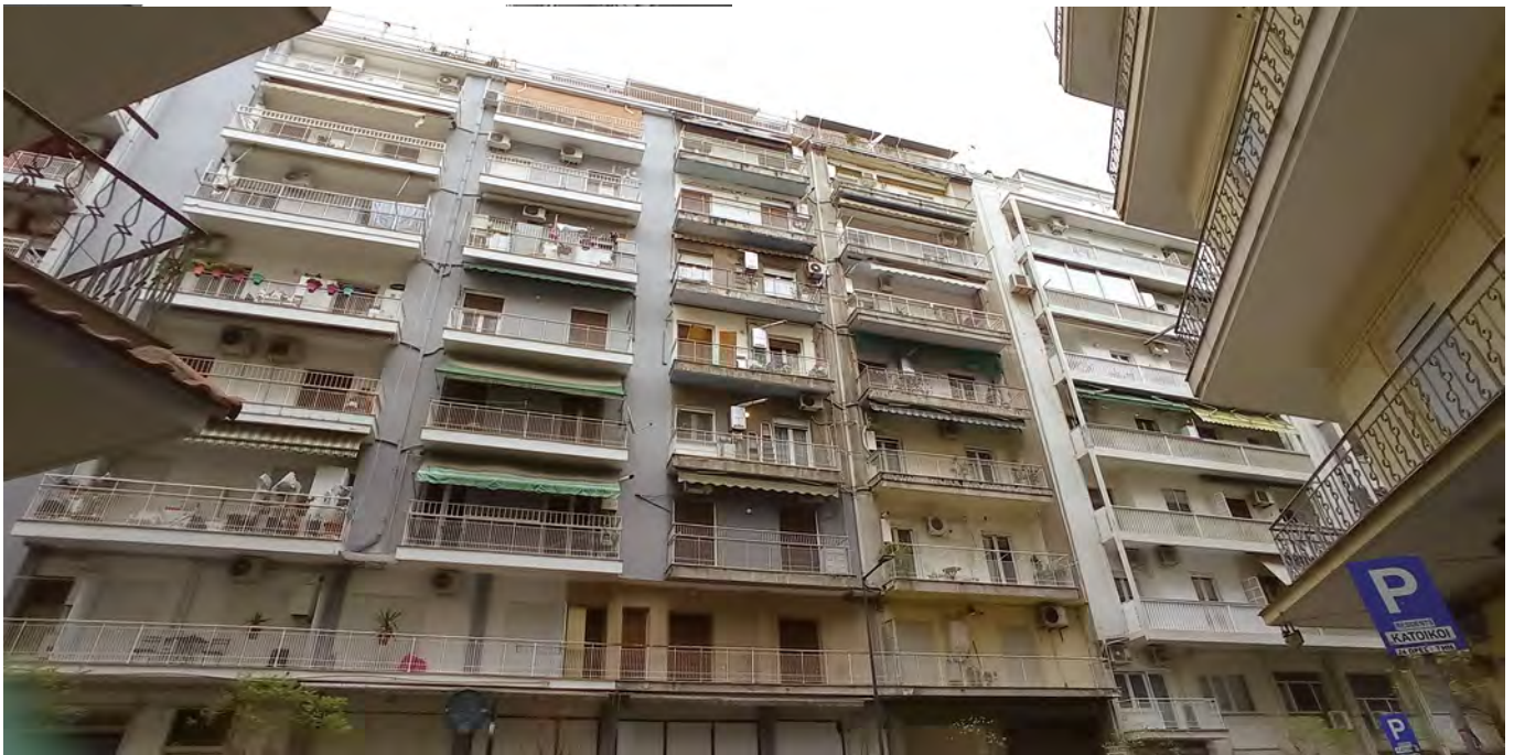
03 The patchwork of individual interventions on the facades. © Sotiria Alexiadou, 2022.
