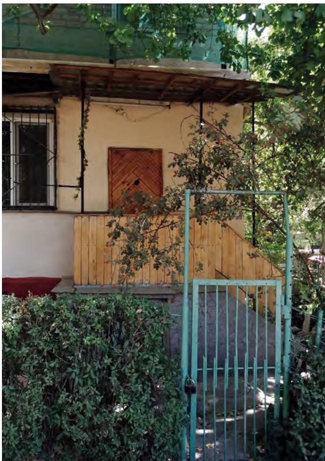
08 Self-adaptation of the ground floor of one of the Soviet housing series with the organization of a separate entrance to the apartment, taking over part of the adjacent communal territory, and rearrangement of the balcony. (Tashkent, YunusAbad -14). © E. Gladkova, 2022.
