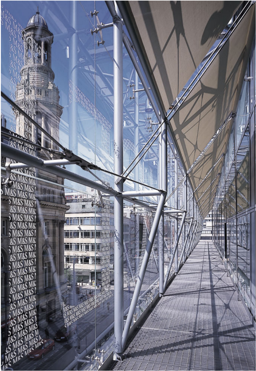
Fig. 5.13 BDP, Marks & Spencer Store, Manchester. Planar construction of the external skin of glass panes supported by regulated brackets, which are assembled to the frame through related profile branches up to the secondary load-bearing structure and accommodate the point jointing devices ( rotulle type). © Courtesy of Charlotte Wood Photography
