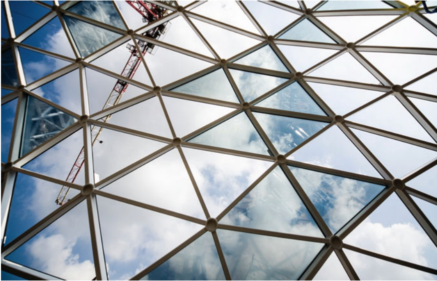
Fig. 3.3 Massimiliano and Doria Fuchs, Roofing System of ex Unione Militare Building, Rome. Construction of the “cloud” on the roof plane according to the connection interfaces between the profile rods supporting the structural silicone connections of the triangular glass enclosure panels. © Courtesy of Pichler Projects
