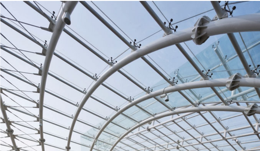
Fig. 5.8 Francesco Cocco, People Mover , “Tronchetto” and “Piazzale Roma” Stations, Venice. Pillars supporting the spherical joints from which the diagonal struts branch off to the transverse struts, on which the couplings for the parallel attachment of the upper tubular beams are set: above the spherical joints the pin for the assembly of the beams is applied, on which the connection of the rotulles takes place. © Courtesy of Oskar DaRiz
