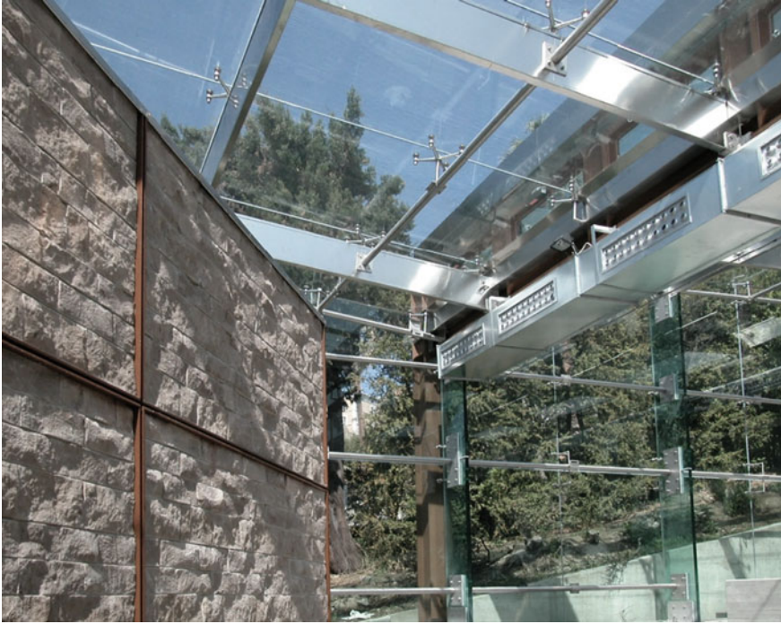
Fig. 5.10 EFA, Collodi Butterfly House , Collodi (Pistoia). Modular glass sheets, to be assembled to the structural grid at multiple connective points (comprising laminated and tempered glass panels for the roof), which are jointed to the vertical blades by means of rotulles designed to transmit the stresses of self-loading, external loads and torsion and bending stresses. © Courtesy of EFA
