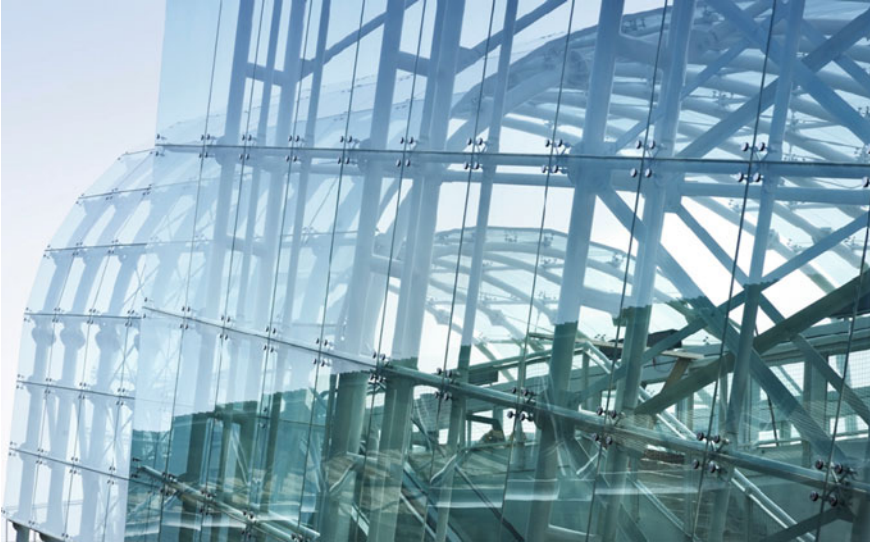
Fig. 5.7 Francesco Cocco, People Mover , “Tronchetto” and “Piazzale Roma” Stations, Venice. Structure with the fixing devices (in spider form) with four or two brackets, depending on the position of use, with the possibility of orbital adjustment. The rotulles have a cylindrical head to be inserted into the drilled and tempered glass modules, equipped with the nylon bushings to avoid direct contact between the metal couplings and the drilled holes. © Courtesy of Oskar DaRiz
