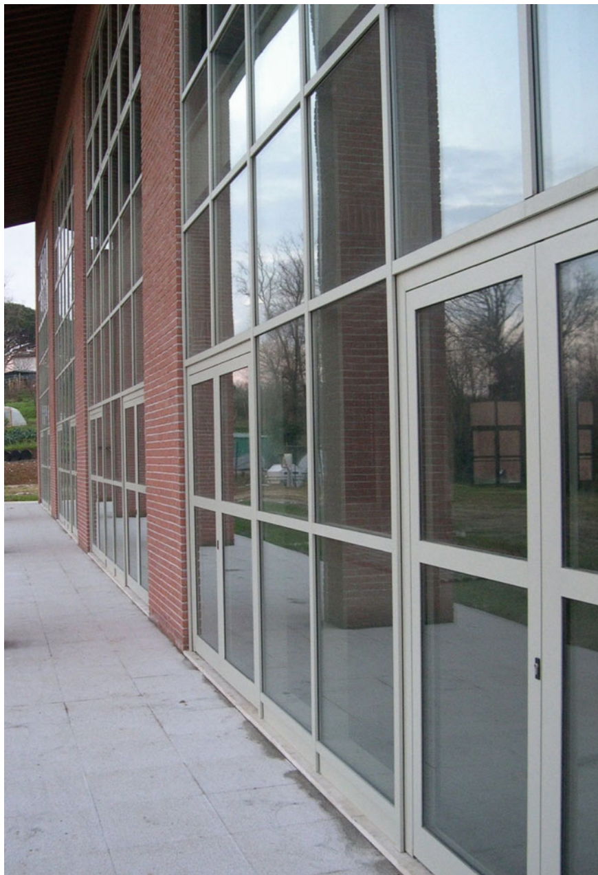
Fig. 2.3 Giuseppe Colucci, School Building, Fauglia (Pisa). Framing of the façade system within the vertical structures, with the interposition of the windows and doors related to the profiles of the homogeneous curtain wall. © Courtesy of Schüco
