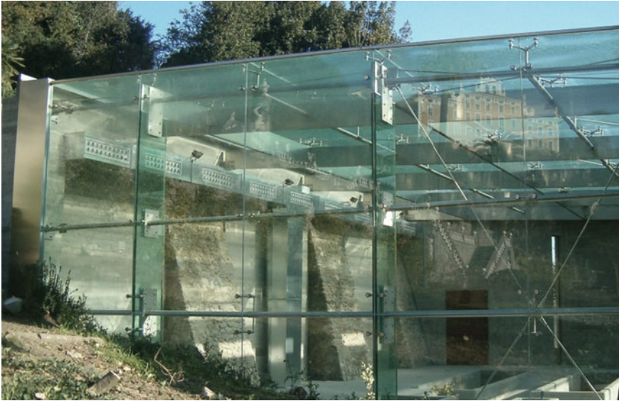
Fig. 5.9 EFA, Collodi Butterfly House , Collodi (Pistoia). Vertical mullions made of glass plates to support the spider-glass joining devices for the mechanical assembly of the glass plates, taking into account the connection of the stainless steel crosses necessary for the attachment of the rotulles (equipped with an internal rotating ball). © Courtesy of EFA
