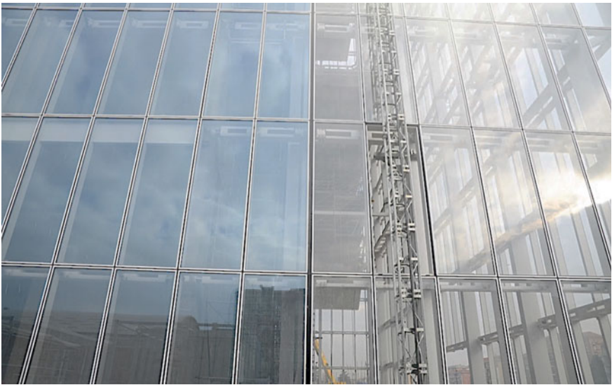
Fig. 4.3 Massimiliano and Doriana Fuksas, Regione Piemonte Headquarters, Turin. Typological and functional sequence of the cellular modules, detecting the detachment with respect to the junction between the different horizontal structures. © Courtesy of Schüco
