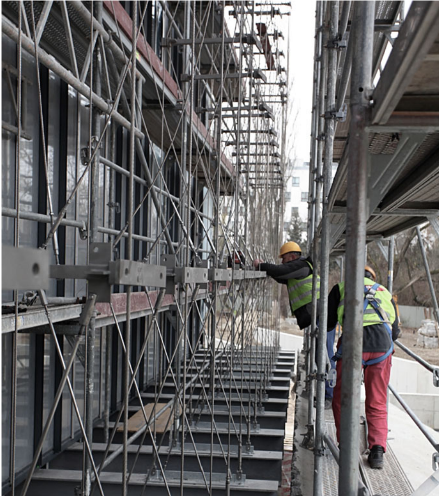
Fig. 5.15 Stelmach & Partners, CSK, Centrum Spotkania Kultur (“Centre for Encountering Cultures”), Lublin. In-situ adjustment of steel segments protruding from the brackets to support spacers for mechanical jointing of the fixing devices. © Courtesy of Lilli Systems
