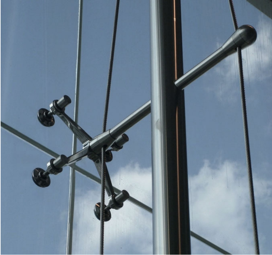
Fig. 5.1 Type of external enclosure composed of tubular profiles supporting steel crosses: these connect the steel rotulles (consisting of a cylindrical body, inserted into the flared hole in the glass, a threaded spherical-headed axle, a polyethylene washer and a steel washer) for fixing the sheets according to a variety of expressive and executive possibilities. © Courtesy of Faraone Sistemi
