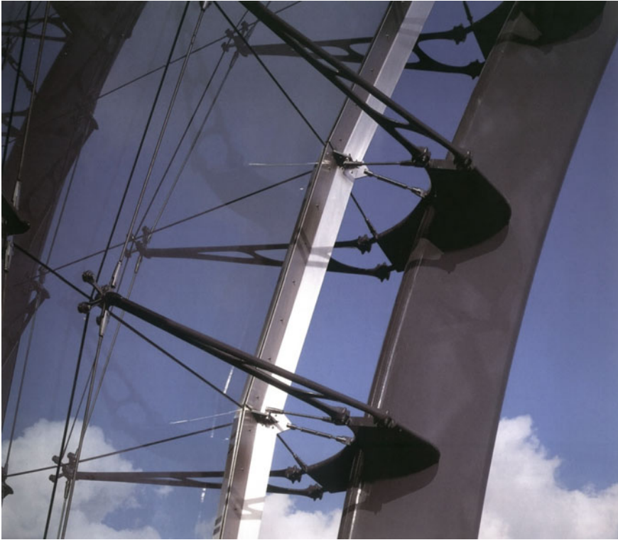
Fig. 5.2 Nicholas Grimshaw and Partners, The Western Morning News , Plymouth (Great Britain). Type of external vertical enclosure composed of the structural apparatus in hollow steel profiles, supporting the brackets (in cast ductile iron) at the ends of which are assembled both the vertical tie rods and the crosses integrated by the articulated bolts for fixing the glazed sheets. © Courtesy of Nicholas Grimshaw and Partners
