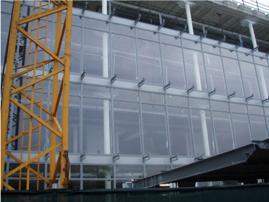
Fig. 4.1 Maurizio Varratta, iGuzzini Lab , Recanati. Assembly sequences of the prefabricated cellular façade components through the mechanical connections of the complete modules to the horizontal structures. © Courtesy of Pichler Projects
