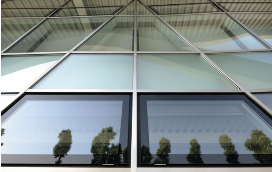
Fig. 2.1 Seiv Group, Sidi Sport Headquarters, Maser (Treviso). Modulation of the mullions and transoms façade system according to the application of the glazing fixing devices and the overlapping of the cladding boards. © Courtesy of Schüco
