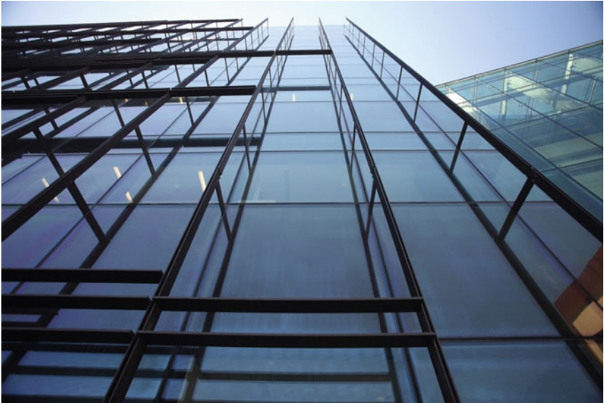
Fig. 3.2 EFA, Chiesi Farmaceutici Headquarters , Parma. Façade system completely planar and without external profiles, while the modules are framed by silicone joints and external rebate gaskets between the frame profiles. © Courtesy of EFA
