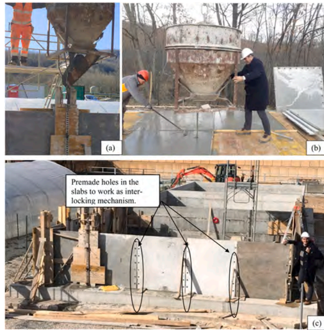
Fig. 4. Construction steps of the third basin – (a): pre-casting the slabs horizontally, (b) cast in place the columns, (c) arranging the precast slabs vertically in their positions before casting the stiffening column.
