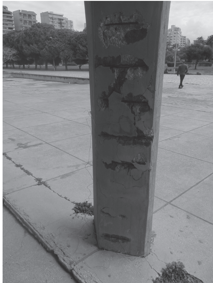
Fig. 4. Oscar Niemeyer, Lebanese pavilion column conditions in 2019. © Joe Zaatar
