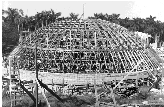
Figure 4. Theatre dome under construction, with scaffolding and wooden formwork visible. Courtesy of ISA archives.
