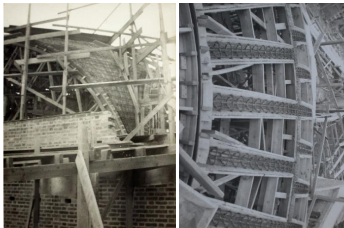
Figure 3. Rebar in the Classroom pendentives (left) and the domes' ribs and rings (right). Courtesy of ISA archives.
