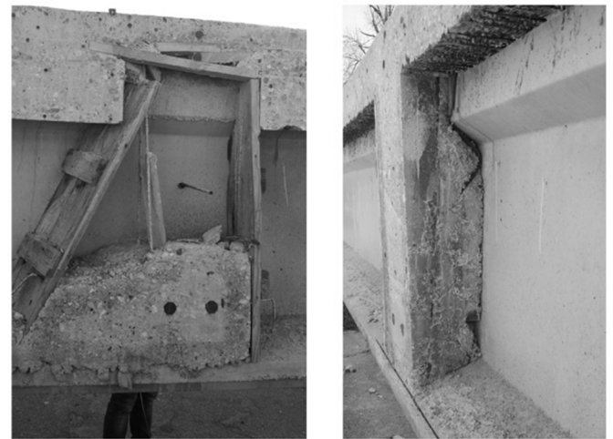
Figure 10. Photos of the cast-in-place transversal beams of two precast beams after the dismantling.
