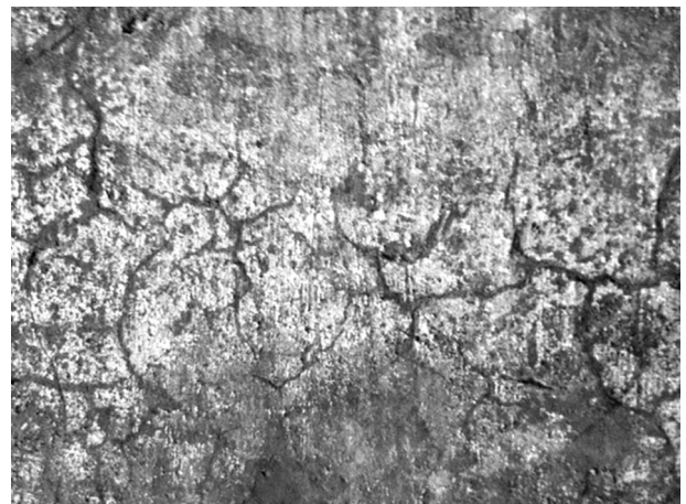
Fig. 6. Sample 1. White efflorescence analysed by X Ray diffraction (see Fig. 7).
