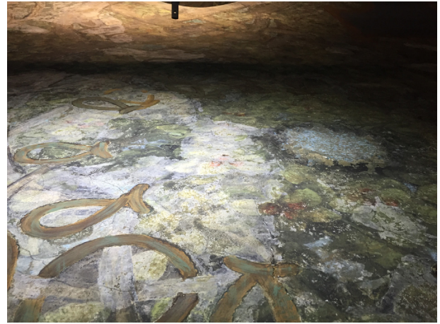
Fig. 4. Polychrome vault: white efflorescences are unevenly distributed forming a whitish covering layer.
