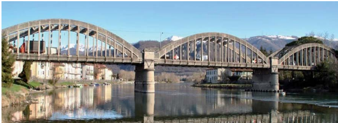
Fig. 1. The Brivio bridge: view from the downstream of Adda River on the Lecco side.
