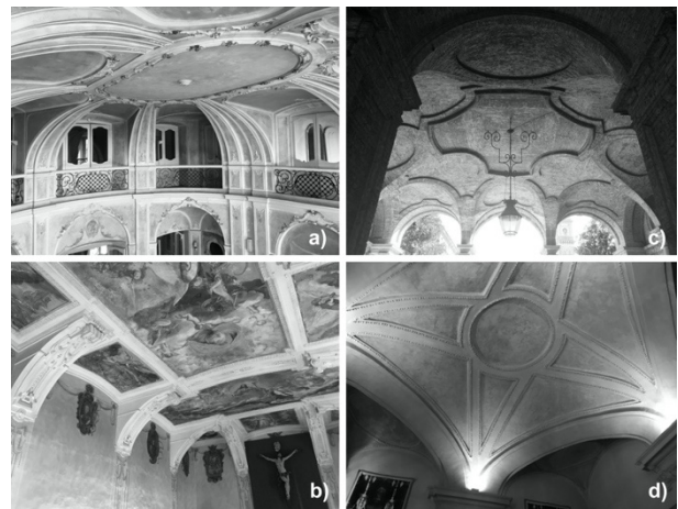
Figure 3: Study of typologies of cloister vaults: a) frame vault of Villa d'Adda-Borromeo, arch. F. Croce (ca. 1765), Cassano d'Adda; b) frame vault of St. Sigismondo refectory (ca. 1758), Cremona; c) planterian vault, Palazzo Ghilini, arch. B. Alfieri (1732), Alessandria; d) a fasce vault, St. Lorenzo church sacresty, arch. G. Guarini (ca. 1680).
