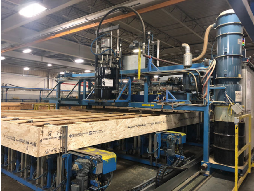
Fig. 5.1 The timber construction industry is an example of the 4.0 revolution: here the prefabrication potential is maximised, starting from the first sawing processes moved to factory decades ago, to the development of CNC assembling processes. Source Author's photo credit at HOME TECHNOLOGY plant, October 2018
