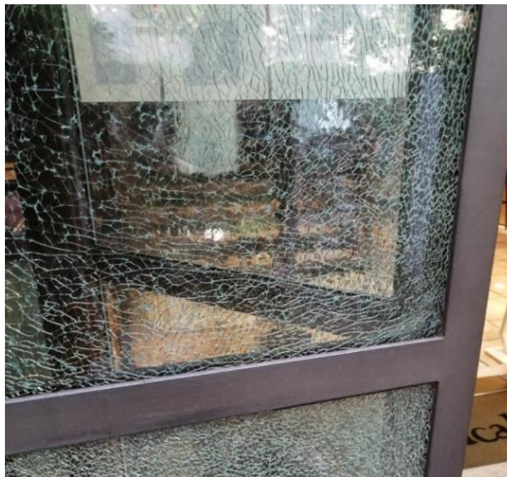
Figure 1. Fractured laminated tempered glass.
