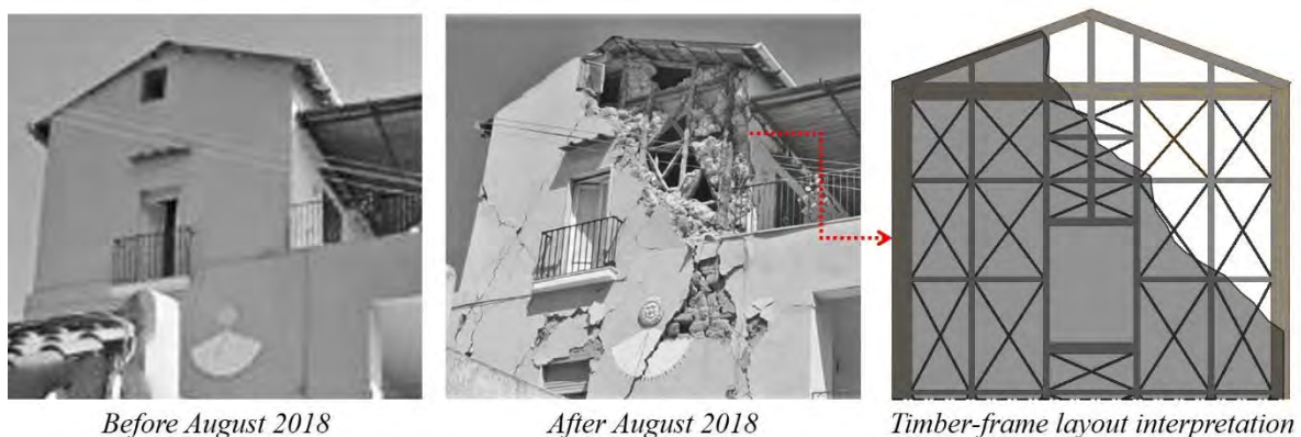
Figure 6: A timber-frame realized in a masonry wall of a house hit by the 2018 Ischia earthquake (representation realized by the authors).
