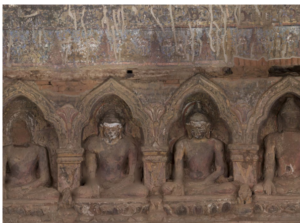
Figure 5. The 2018 orthophoto of the East inner wall in Myin-pya-gu. Areas of the image are out of focus and unevenly lit with shadows in the Buddha niches (Credit: © Carleton Immersive Media Studio; Carleton University).
