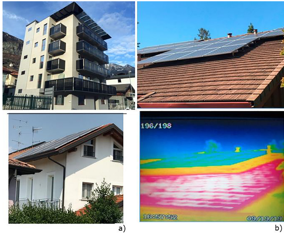
Fig. 2. a) Examples of rooftop PV systems in existing buildings in Northern Italy (Images acquired by D. D'Agostino); b) Visible and IR image illustrating impact of shading from photovoltaics on thermal heat gain to brown tile roof. Colour is proportional to temperature, with white and red hottest, and black and blue coolest (Comparative image and thermograph by D. Parker). (For interpretation of the references to colour in this figure legend, the reader is referred to the web version of this article).
