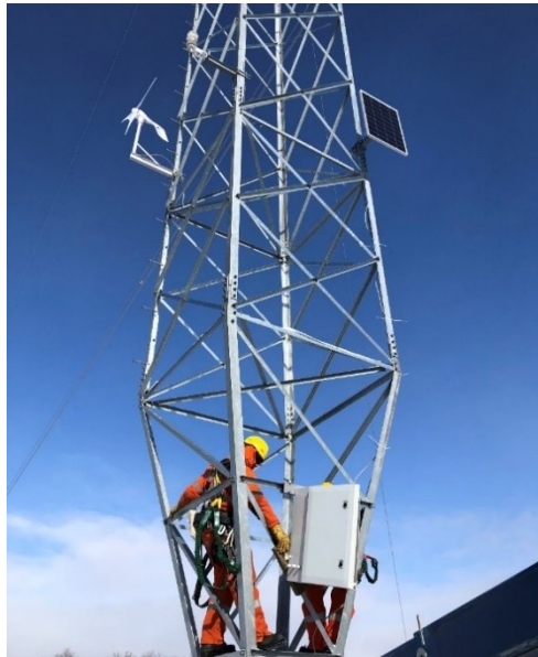
Figure 3 – Arrangement of the base station on the lattice structure of the tower
