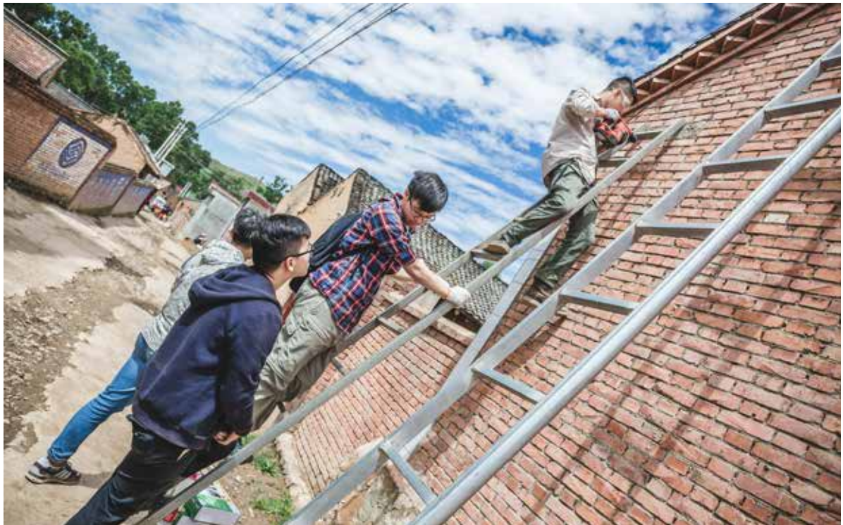
Figures 4-6 (pages 113-117): Light for the village (2017): Installation of solar light panels and village improvement projects in Datan Village, Zhangjia County, Gansu, China. Source: author.
