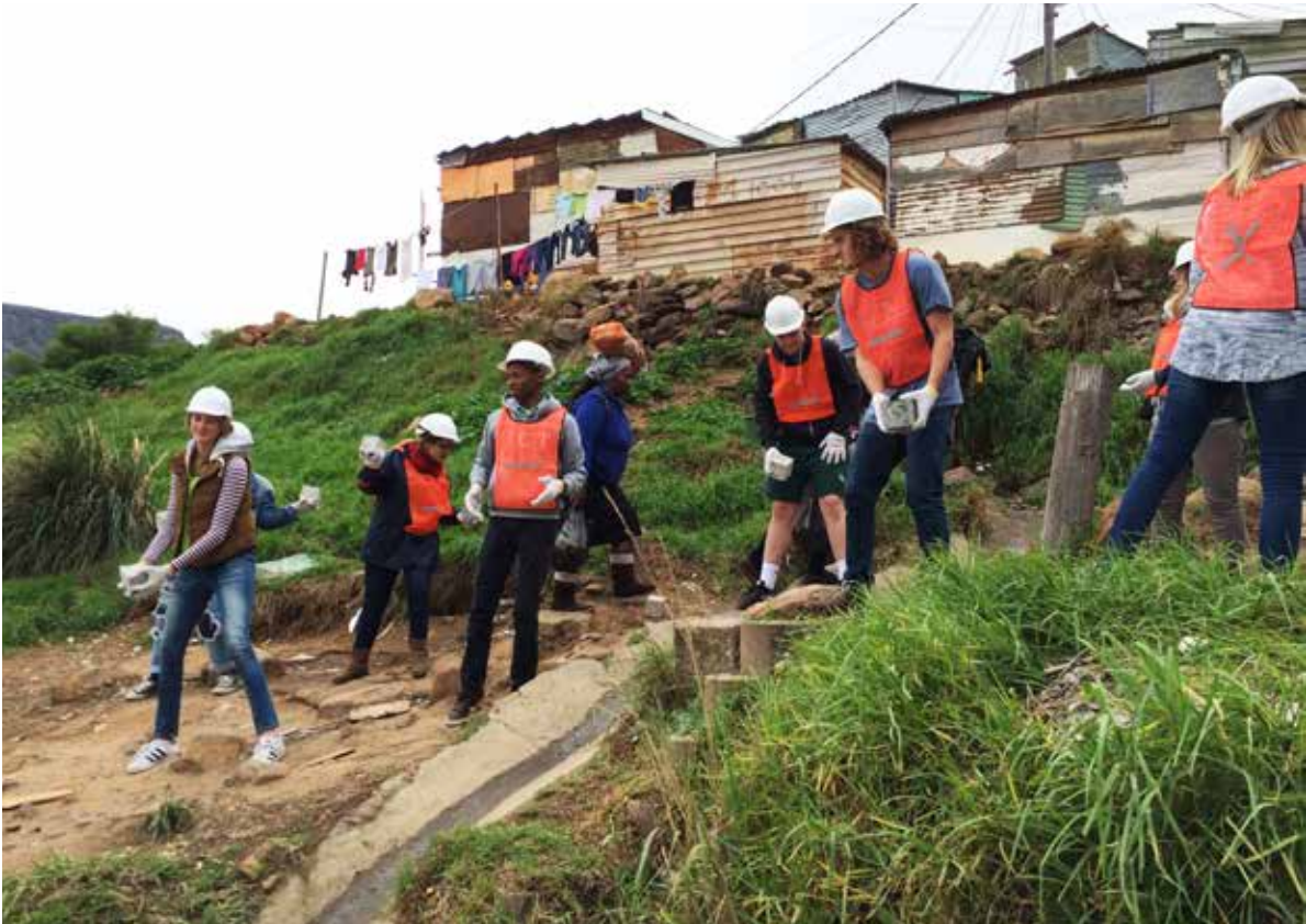
Figure 3 (page 37, top): Students assembling the formwork for the staircase that leads up to the 2012 water platform from O.R. Tambo Road in Imizamo Yethu. Source: author
