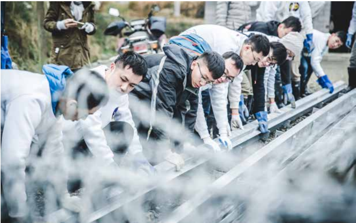
Figures 1–3 (pages 110–112): Feungshan Village, Wu Zhi Qiao (Bridge to China) (2017): Gabion bridge design and build in Feungshan Village, Qianjiang District, Chongqing, China. Source: author.
