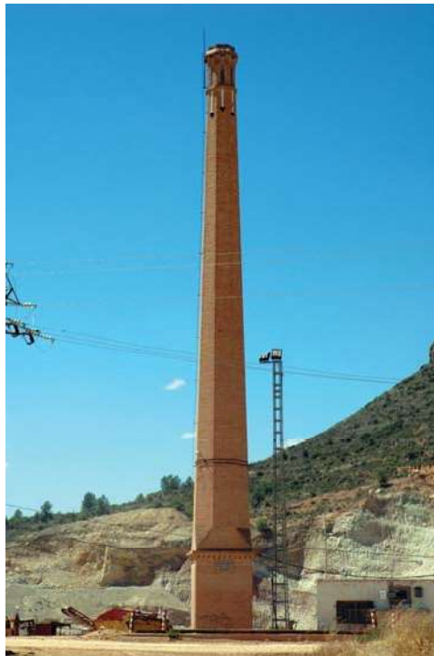
Figure 1: The chimney located in Villar del Arzobispo (Spain) used as a case-study of this research.
