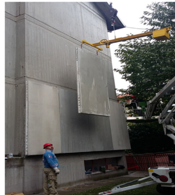
b) Panel's assembly in parallel to the line of the façade via rocker
