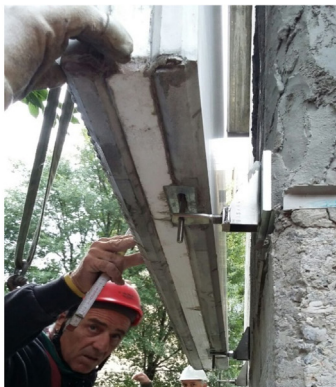
c) Panel's positioning through inclusion in the boxes of the panels of the facade on the HALFEN pins
