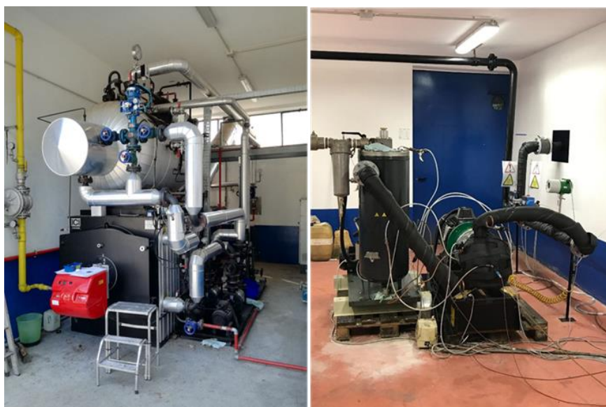
Figure 1. Steam generator area (left) and expander area (right) of the test rig employed in this work.
