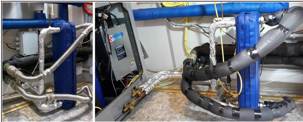
(c) Plate heat exchanger between the heat pump and the "intermediate-temperature" tank
