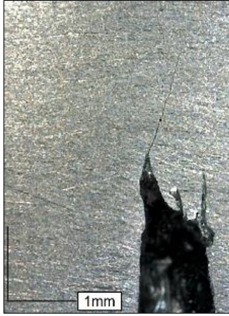
Fig. 6. Crack nucleation from the notch at the rivet hole.
