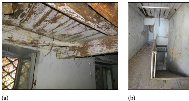
Fig. 15. Timber floors were present at all story levels both in (a) the Italian (image by Nicola Ruggieri); and (b) the Greek tradition (image by Sandra Tonna).
