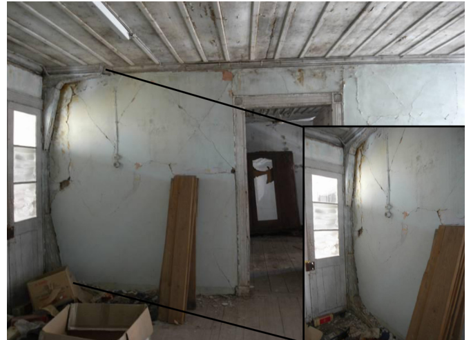
Fig. 9. Timber columns along the external wall. Details of the two curved reinforcing elements at both corners are shown. (Images by Sandra Tonna.)
