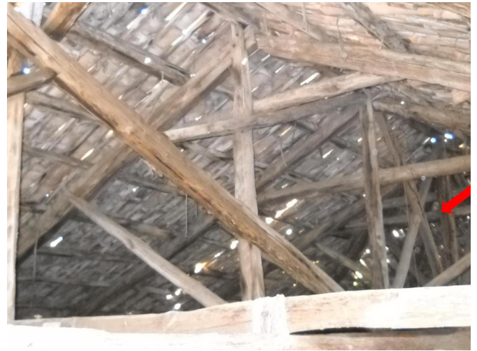
Fig. 14. Timber truss system, characterized by the presence of Saint Andrew's crosses. (Image by Nicola Ruggieri.)
