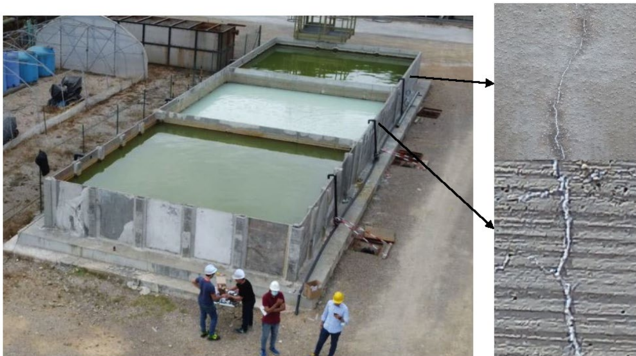
Figure 20. Evidence of crack sealing as monitored during a water filling test of the pilot on 14 May 2021.
