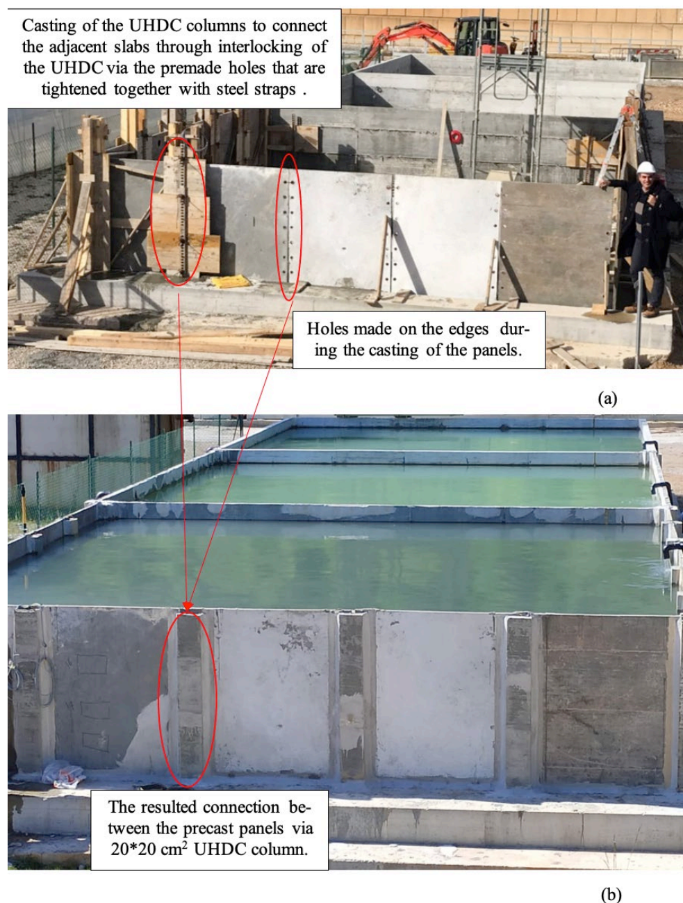
Figure 2. Pictures of the structure, taken on 13 February 2020 (a) and on 20 April 2021 when a full load test was performed filling the three basins (b).
