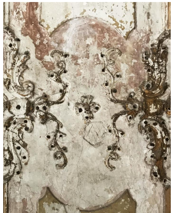
Figure 12. Wall 4: detail of the keying layer and of the iron nails used for on-site made stuccoes.
