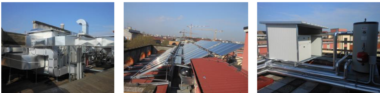
Fig. 1. Photos of the installation, from the left: DEC AHU, solar collector field and the electric heat pump.
