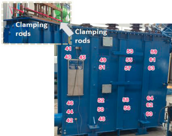
Fig. 1. The 750kVA test transformer. Insets: a detail of the looseness of winding clamping structure (left) and of measurement points (right).
