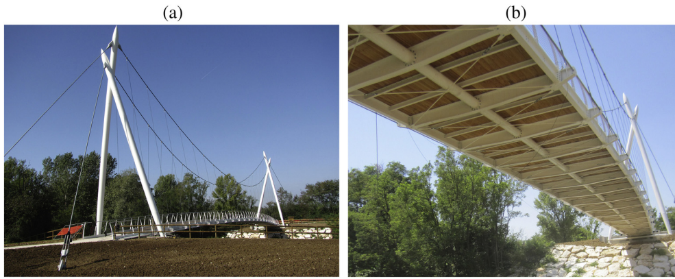
Fig. 1. Footbridge crossing the Serio river (Seriate, Italy): (a) General view; (b) Underside view of the deck.
