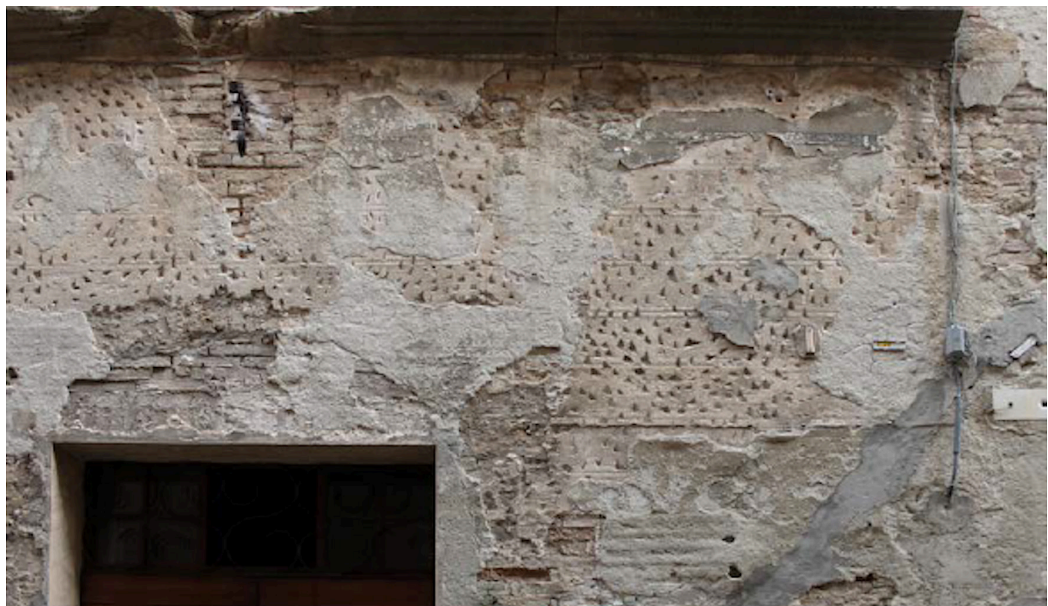
Fig. 9. Pienza, Palazzo Cittadini, graffiti dismantled and tapped (photos by the authors).
