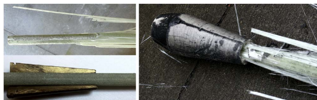
Fig. 3. Failure due to fiber trimming on the collar of the anchor area.
