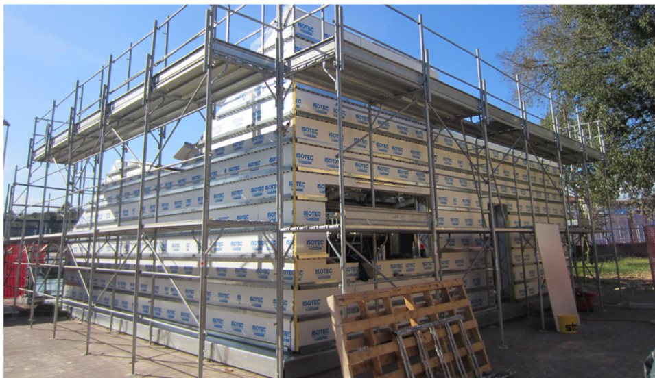
Fig. 16. Image from the construction site. The building is covered with polyurethane panels, which have an in-built horizontal metallic profile for an easy implementation of the cladding with ventilated cavity.
