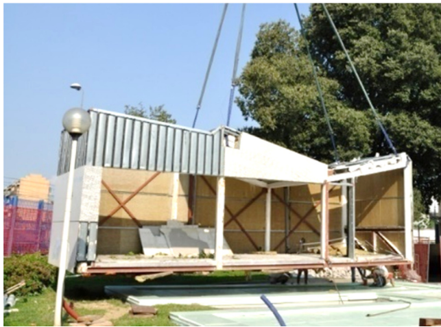
Fig. 2. Atika's prefabricated blocks. The structural modules are kept as the original design of Atika. The core blocks arrived on the construction site pre-assembled and new layers for improving the building's energy efficiency have been added on site. In this picture, the left side of the building is shown, the metallic structure and the internal insulation are visible.
