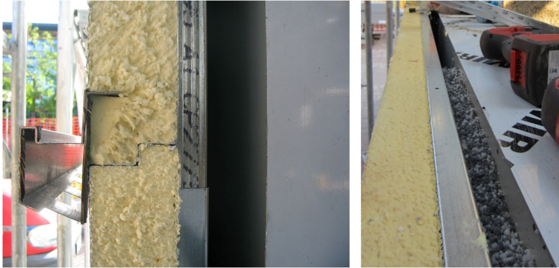
Fig. 18. On the left, gap between the old and the new façade. On the right, the gap filled with powdered insulation.
