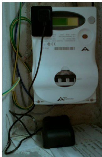
Figure 3. The power meter transmitter for the energy consumption measurement.
