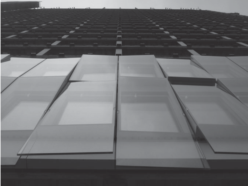
Fig. 8.6 Examination of “multi-layer” systems in order to generate “greenhouse effect”, “chimney effect” and natural ventilation devices in the form of double skin façades. Progetto CMR, Garibaldi Business Centre, Milan © Courtesy of Progetto CMR
