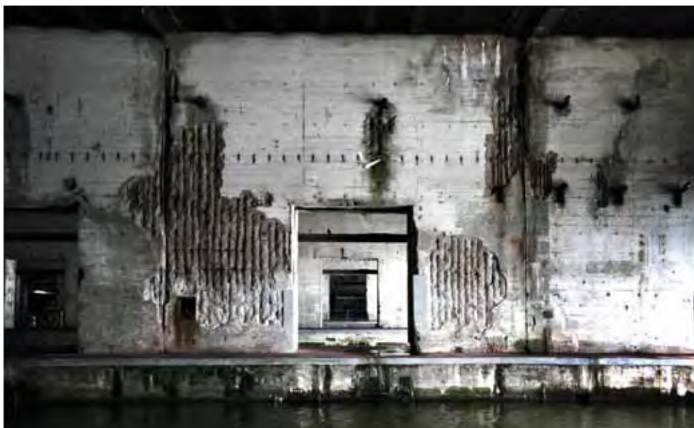
View of one of the interior gateways through the corridors of the bunker. Saint Nazaire (Ph. Claudia Brunelli)
