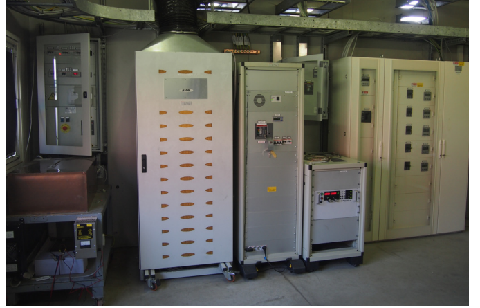
Fig. 6. Photo of the RSE dc microgrid.
