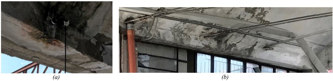
Figure 13 (a) beam T8; (b) beam T1
