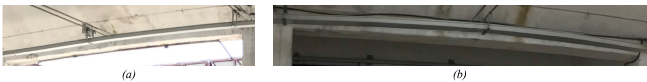
Figure 14 (a) beam T4; (b) beam T15
