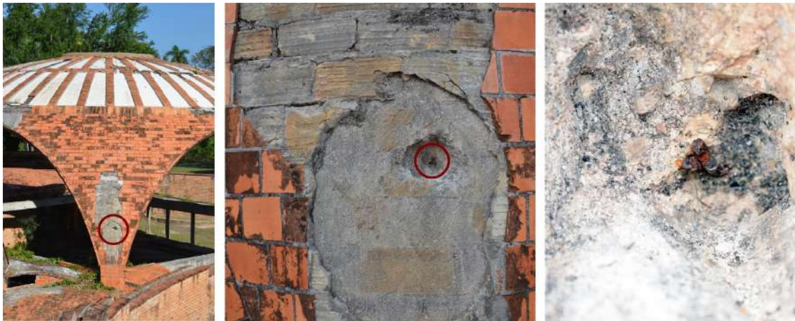
Figure 3. The pendentives of the dance pavilion’s dome. The loss of the outermost layer of tiles unveiled the presence of reinforced concrete. The picture on the right shows the visible tie wire.
