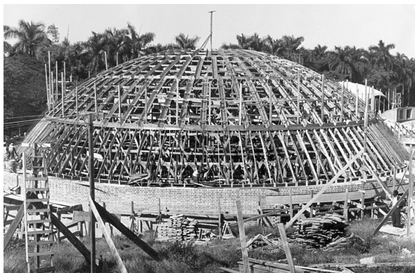
Figure 4. The School of Ballet’s choreography theater during construction. The photograph depicts the wooden formworks for the casting of the dome’s concrete ribs and rings (ISA archive).
