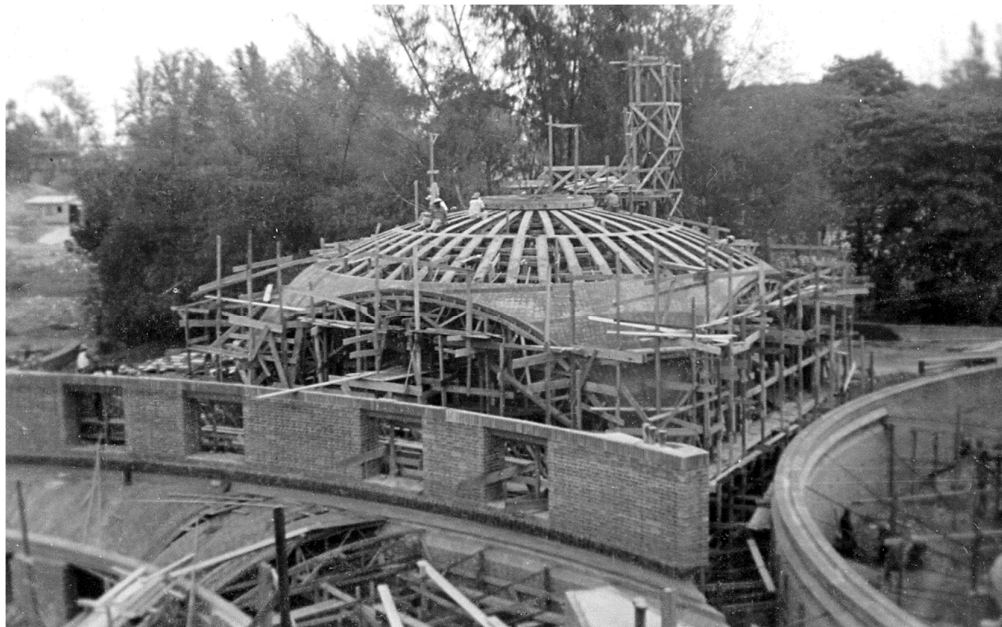
Figure 10. One of the dance pavilions after the concrete casting. The picture clearly shows the concrete framework hidden beneath the current clay tile covering (ISA archive).
