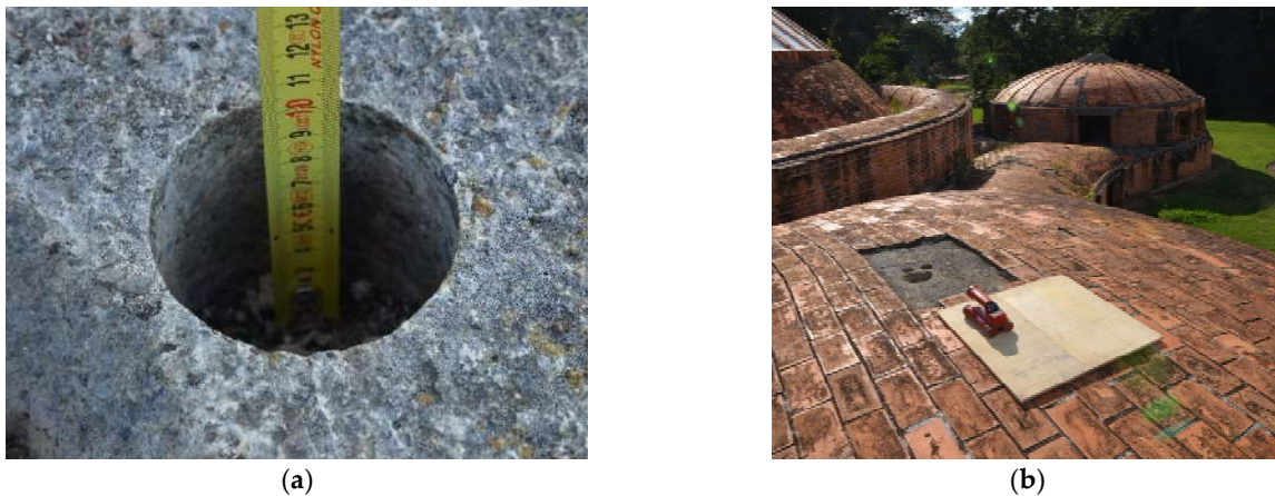
Figure 16. (a) The 10 cm hole left by previous core testing, proving the presence of a concrete slab (photos by the authors). (b) Pachometer testing performed to detect possible rebar in the same vault.
