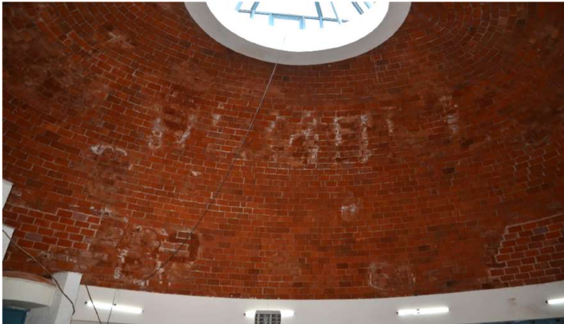
Figure 26. Efflorescence patterns at the intrados of the domed classrooms (photo by the authors).
