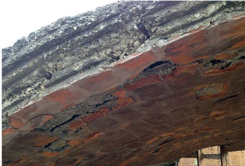
Figure 23. One of the vaults replaced with plain concrete vaults. The poor quality of the materials employed resulted in delamination and consequent exposure of steel rebar (photo by Luca Valisi).
