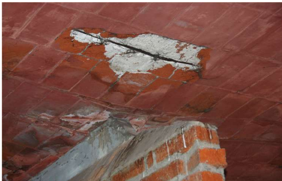
Figure 19. Exposed steel rebar at the intrados of the pasillo (photograph by the authors).
