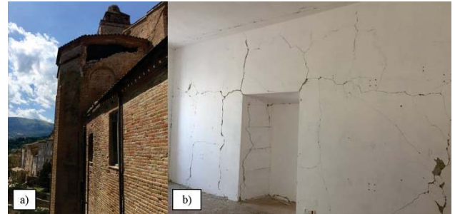
Fig. 3 External cracks on bell-tower and apse a), internal cracks on a wall of the cloister b)
