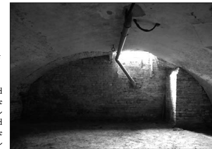
137. In the great cellar corresponding to the hall of the "piano nobile", the northern wall under the façade seems to have been moved towards the street by more than one metre where a portion of barrel vault is separated from the pre-existing one by a fabrication joint.
