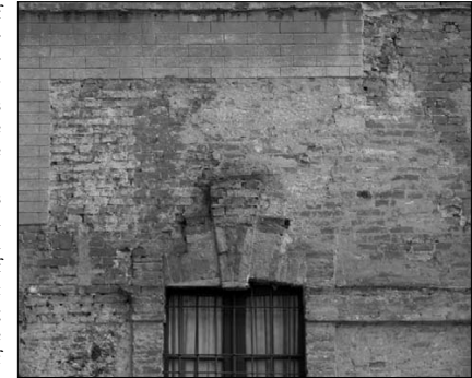
134. The fascia which connects the window frames to each other on the ground floor is realized in brick limited to the median tract of the façade. In the lateral tracts corresponding to casa Lotica and the house belonging to Ferrante Magio, the fascia is formed with a "rincoccio" and secured to the underlying brickwork (M 3 ) with nails which are still partly visible.
