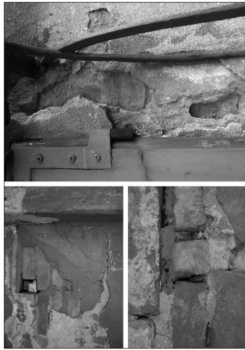
141. Clay appears as a constituent of almost all the plaster mortars on the façade and the bedding mortars of Palazzo Magio Grasselli where it was used to bind both fired and unfired bricks.
