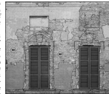
131-132. Map of the stratigraphic units of the façade of Palazzo Magio Grasselli: a general table and details of the twelfth and thirteenth windows on the "piano nobile".
