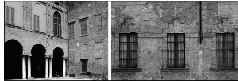
136. In the median tract of the façade, a solution of horizontal continuity distinguishes the brickwork in brick and lime mortar with window frames in phase with the ground floor of the overhanging brickwork and mortar of "bazzana" which forms the "piano nobile" and the frames. The same discontinuity is also found on the two courtyard façades, suggesting an intentional construction choice rather than a contingent heterogeneity of materials during the 17th century building site.
