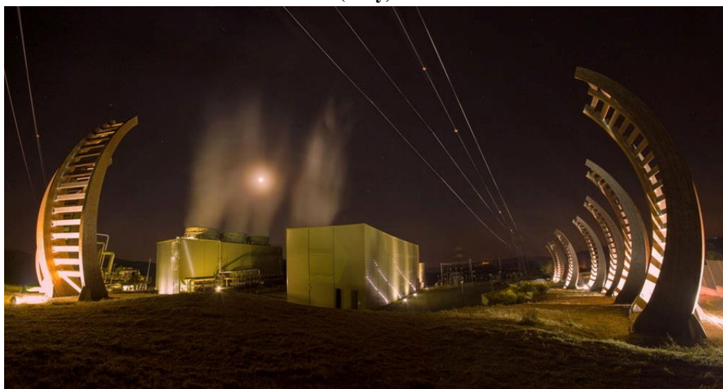
Figure 5 – Geothermal and Biomass integrated plant in Castelnuovo Val di Cecina (Italy).
