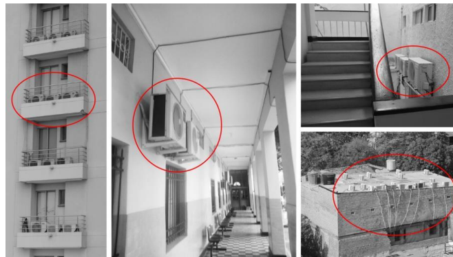
Figure 2. Example of balconies and other spaces used to house air conditioning equipment.
