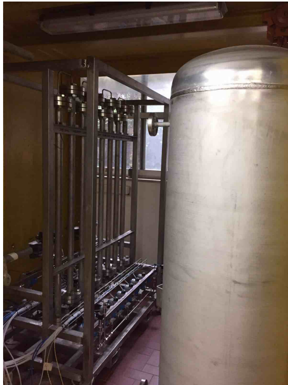
Fig. 5. Test plant used for characterizing and selecting sorbents for the UAr extraction plant PSA unit.
