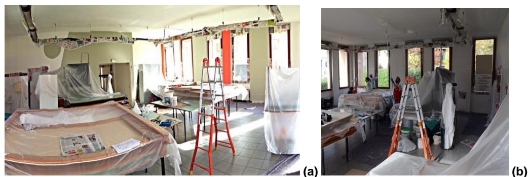
Figure 1. The renovation of the civic center: (a) the civic center (b) citizens at work
